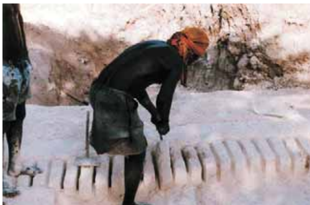
Figure-5: Workers and coral lime stones mining techniques in Manda Island, Lamu archipelago, Kenya Source: S. Pradines
