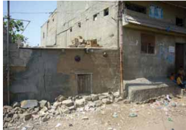
Figures 12: A house foundation sinking in Machar Colony
