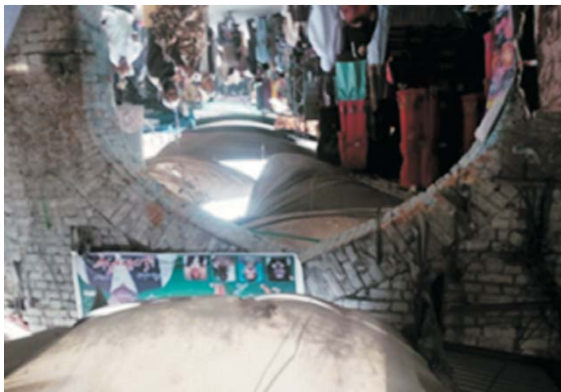
Figure 16a,b: Existing condition of main entrance gate of Shahjehani Sarai.
