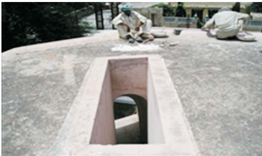
Figure 12a,b: Roof top of the tomb before and after renovation (Government of Punjab, 2012).
