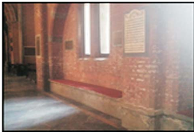
Figure-13: The northern interior wall affected by dampness.
