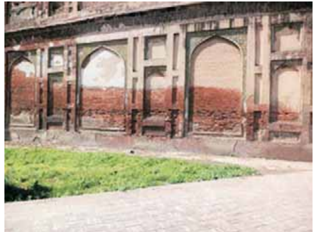
Figure-3: Dampness on brick wall.
