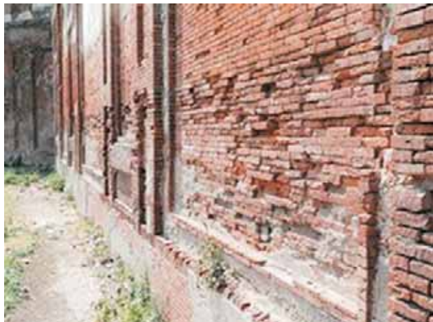
Figure-4: Erosion of mortar from brick wall.
