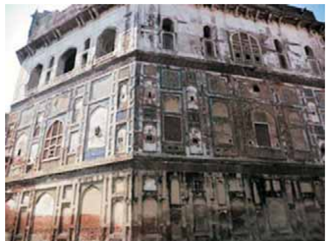
Figure-8: Neglect of wall of Shish Mahal
