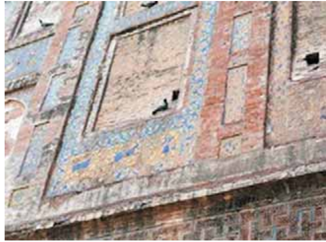
Figure-10: Destruction due to pigeons
