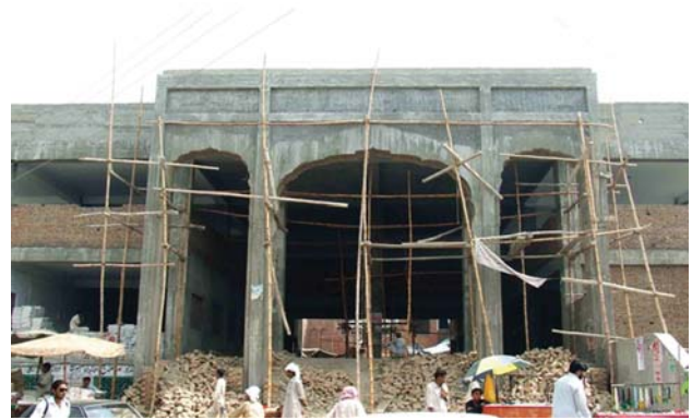
Figure-3: Newly constructed Entrance from Sahiwal Road to the shrine of Bābā Farid.
