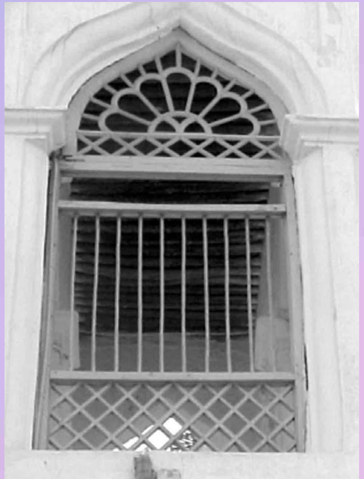
An opening on a seafront house in Sur Lawati the traditional trading quarter.
